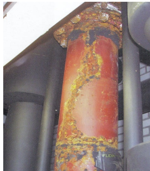
Fig.5 Example: stress crack corrosion
